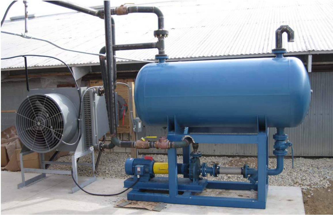
Hot Oil System and Fan Coil Ducted Into House
